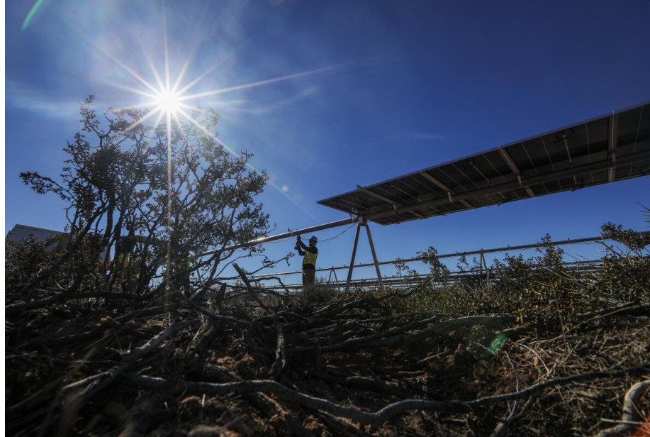
A construction worker pulls wiring at the site of the Gemini solar farm, on public lands outside Las Vegas, in January 2023. (Brian van der Brug / Los Angeles Times)
